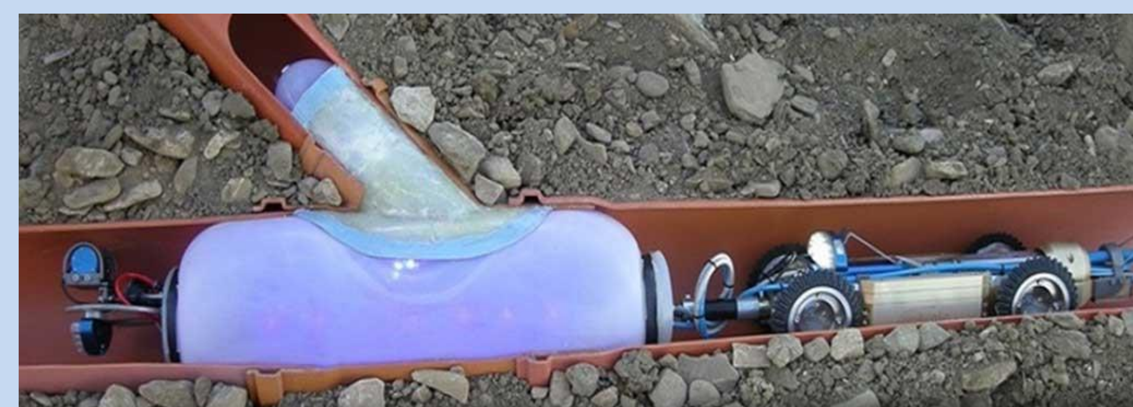
Top Hat (installed at lateral-main connection to provide leak proof
