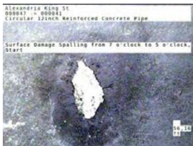
Spalling damage of pipe surface
