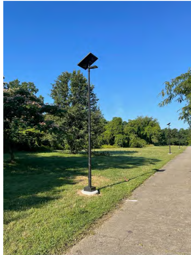
Ben Brenman Park solar lighting
