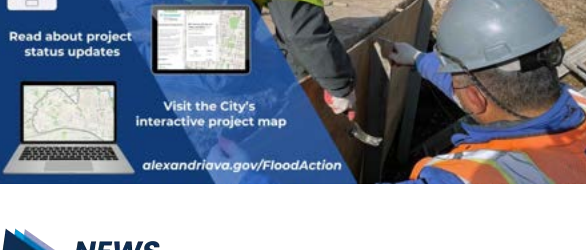
Crews work to build a new environmentally friendly retaining wall along Timber Branch.
