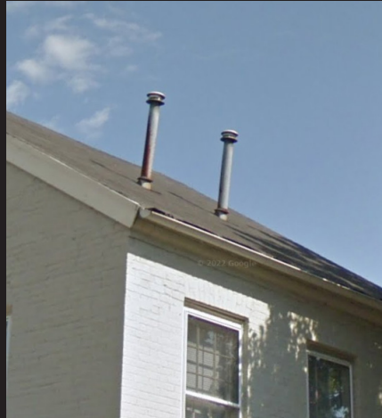
Example of an inappropriate exterior metal flue chimney on a historic building.
