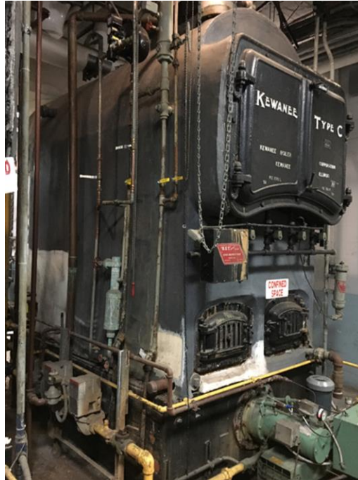
Converted City Hall boiler
