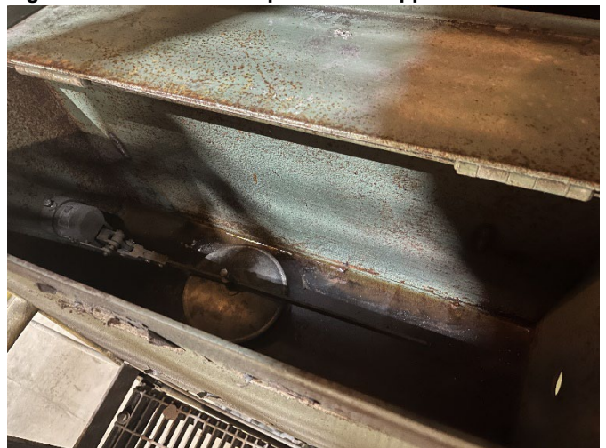
Figure 16: Boiler No. 2 Full Water Level Box.
