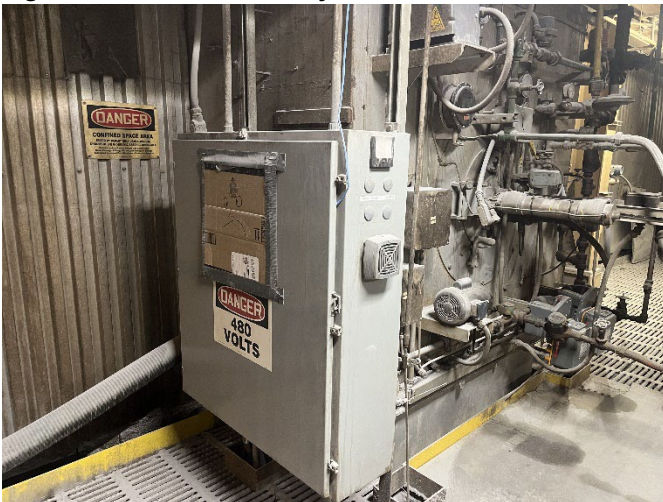
Figure 21: Boiler No. 2 Auxiliary Burner Control Panel.
