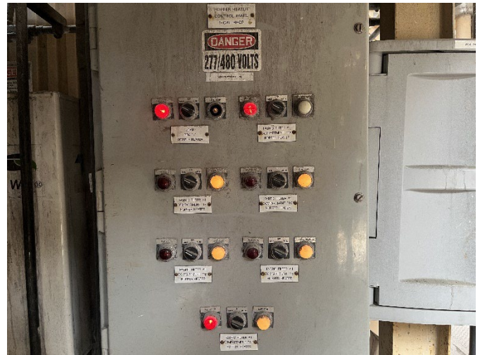
Figure 28: Baghouse Hopper Heater Controls Set To Manual. Punchlist Item Since 2021.
