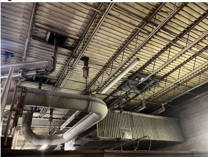
Figure 23: Lights Not In Service Over Boiler No. 2.
