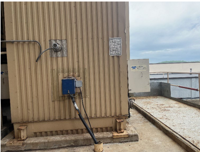
Figure 29: Baghouse No. 3 Opacity System Installed.
