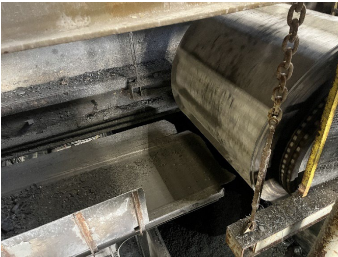
Figure 9: Ferrous Drum Magnet In Operation.
