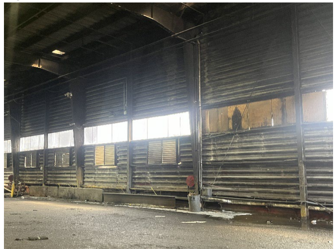
Figure 6: Dirty And Damaged Walls In Tipping Hall.
