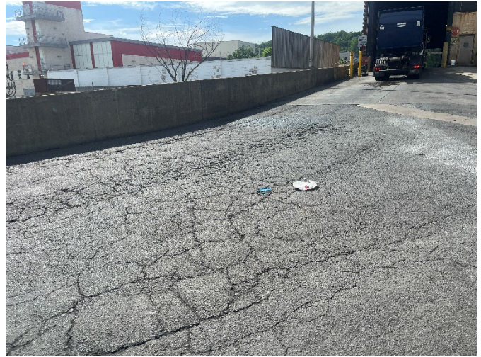
Figure 2: Pavement Spider Cracking At Tipping Floor Entrance. Punchlist Item Since 2016.
