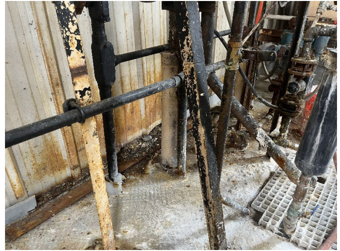
Figure 26: Deterioration Behind Lime Slurry Piping Of SDA No. 2. Punchlist item since 2019
