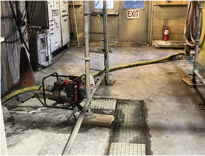
Figure 7: Temporary Pump set up to transport wastewater from the trench drains to the Cooling Tower basin. Punchlist item since 2022.
