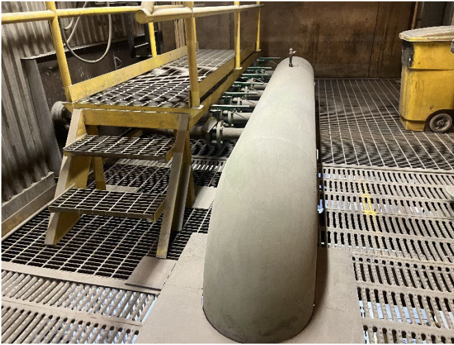
Figure 19: Boiler No. 1 LN System.
