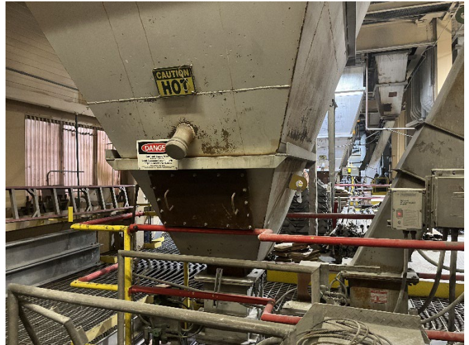
Figure 14: Boiler No. 1 Superheater Hopper.
