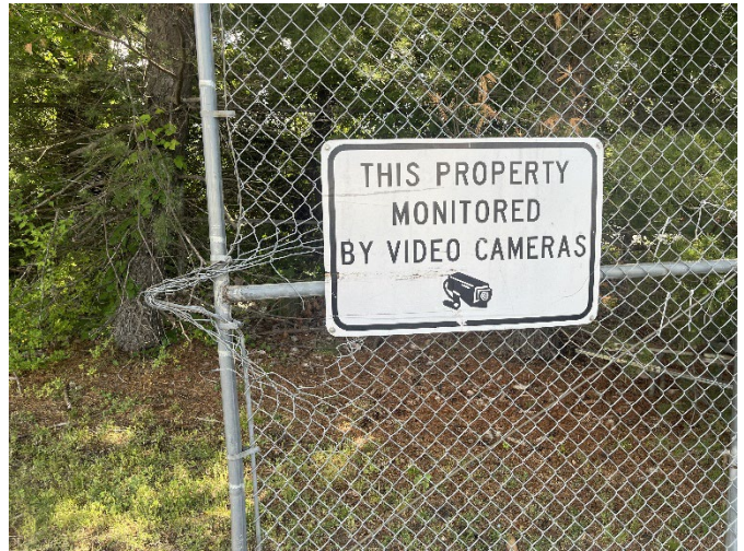
Figure 4: Entrance Gate Wire Pulled Apart.
