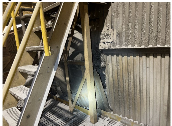
Figure 24: Insulation Deteriorating Around Boiler No. 3 Steam Drum. Punchlist Item Since 2021.
