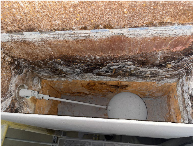
Figure 13: Boiler No. 1 Water Box Empty.
