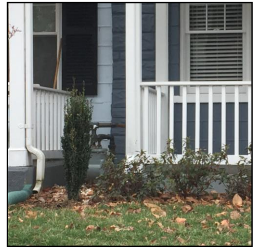
Meter may be located on the façade between porches. Paint meter to match the adjacent wall color.
