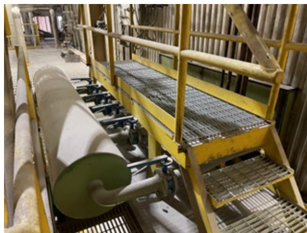
Photo: New LN equipment on Boiler No. 3 as part of the Low NOx Technology Installation
