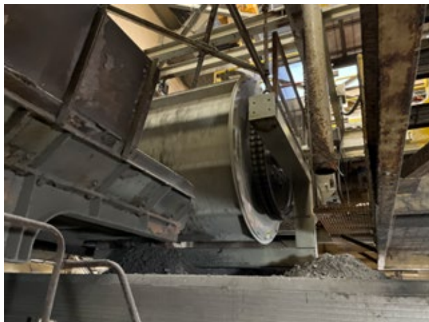
Photo: New ferrous magnet installed
