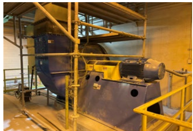
Photo: New LN Fan on Boiler No. 3 as part of the Low NOx Technology Installation.
