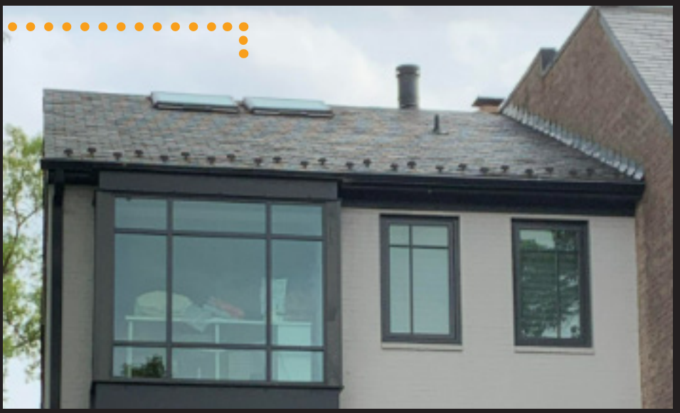
Example of a minimally visible skylight installed on a roof.
